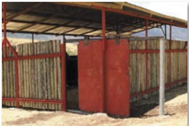
Boma door with beam at top and bottom. Boma walls supported by vertical poles and horizontal channel.
